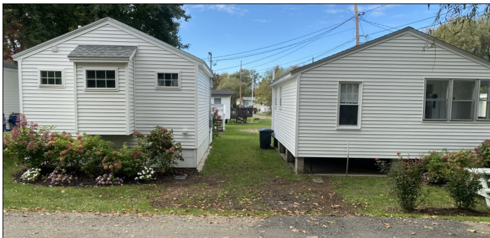
2 new summer line water meters installed for 4 Summer Breeze
