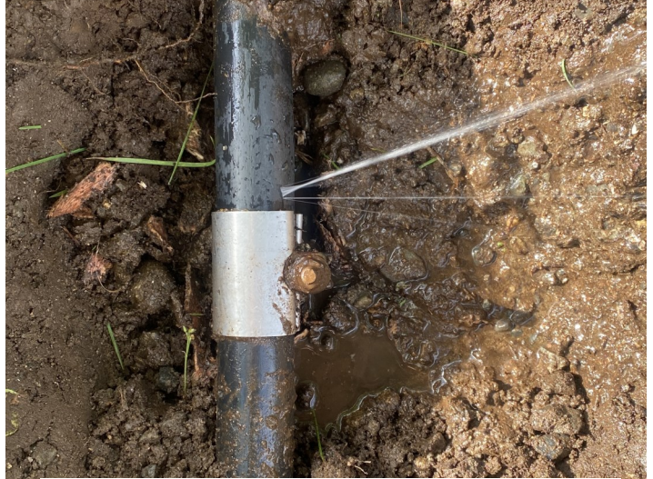
Nicole Rd summer line leak
